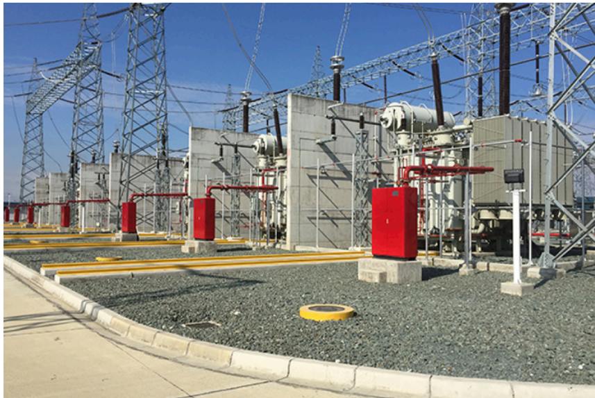
Explosion Prevention and Fire Extinguishing System for Transformers and Reactors
